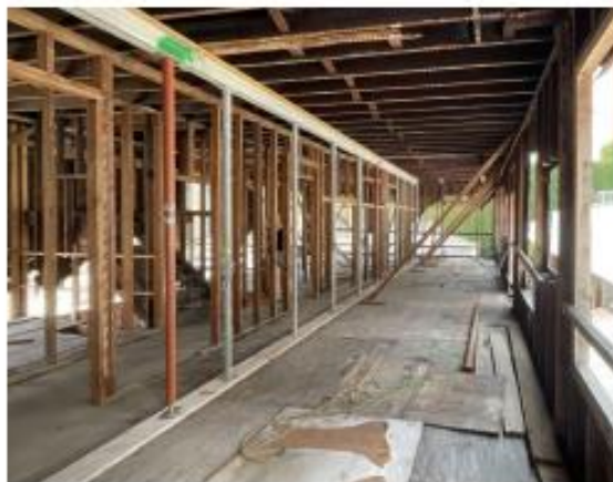
Gutted interior with pieced wood flooring and missing rear wall
