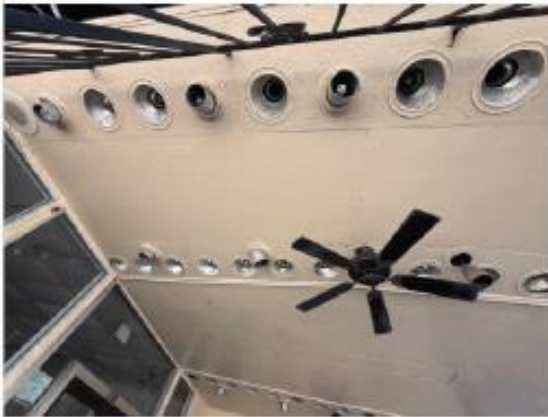
Photo 8: Historic Display Case Lighting
